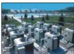
Twelve Heat Siphons installed on Cranberry Twp, PA Community Pool
