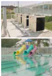
Four Heat Siphons on Fort Lauderdale, FL Community Pool
